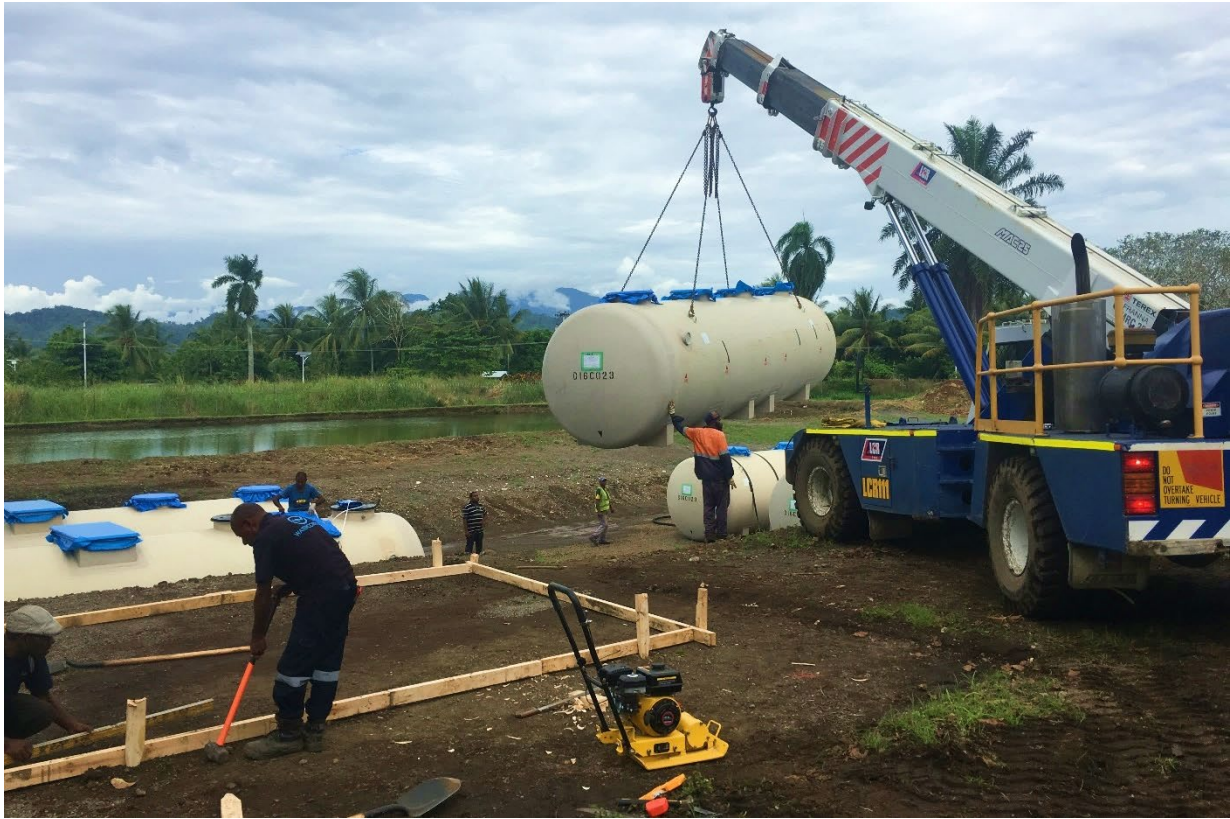
Figure 11 – Collaboration with onsite personnel and local contractors was essential in the smooth installation of the STP.
