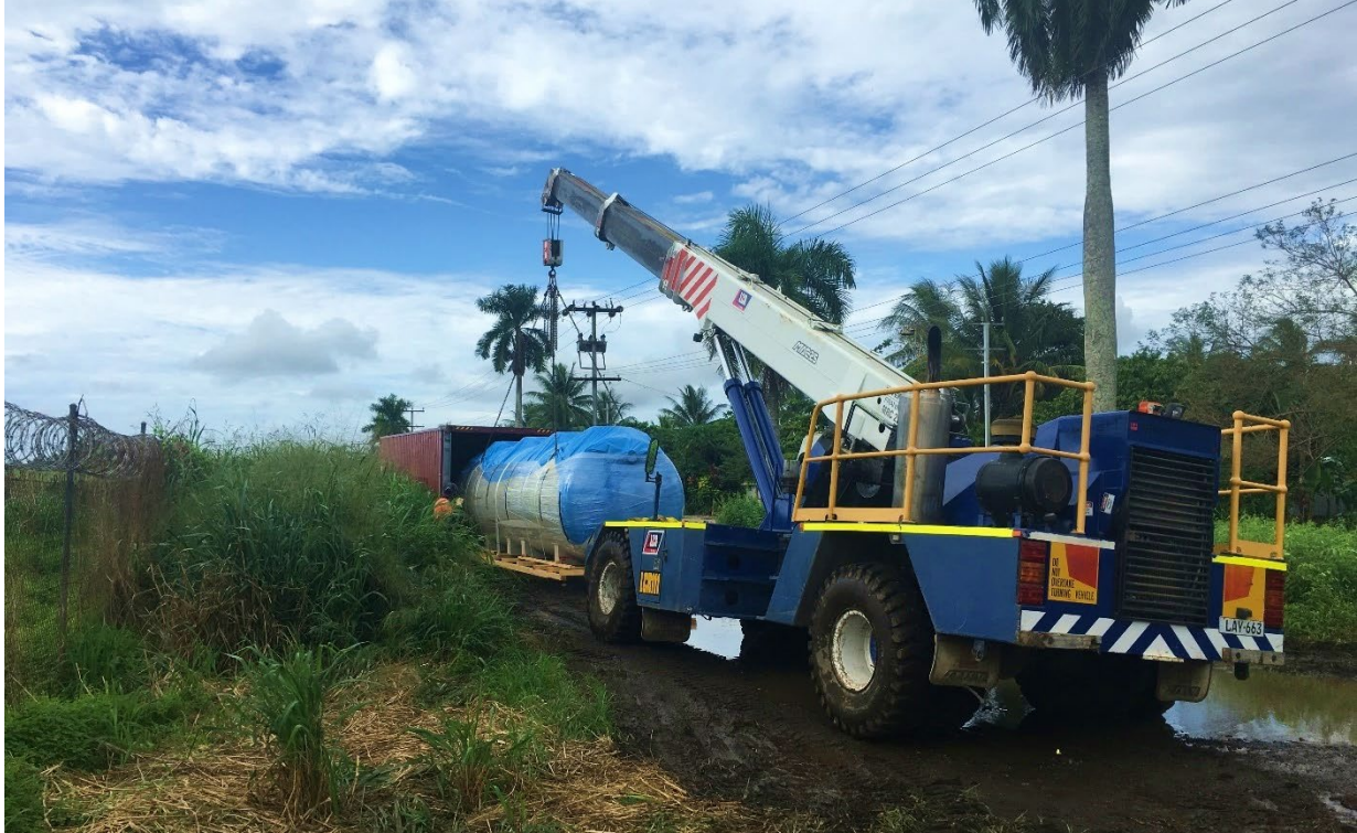
Figure 9 – The Kubota STPs and all components were transported in shipping containers and delivered to site.
