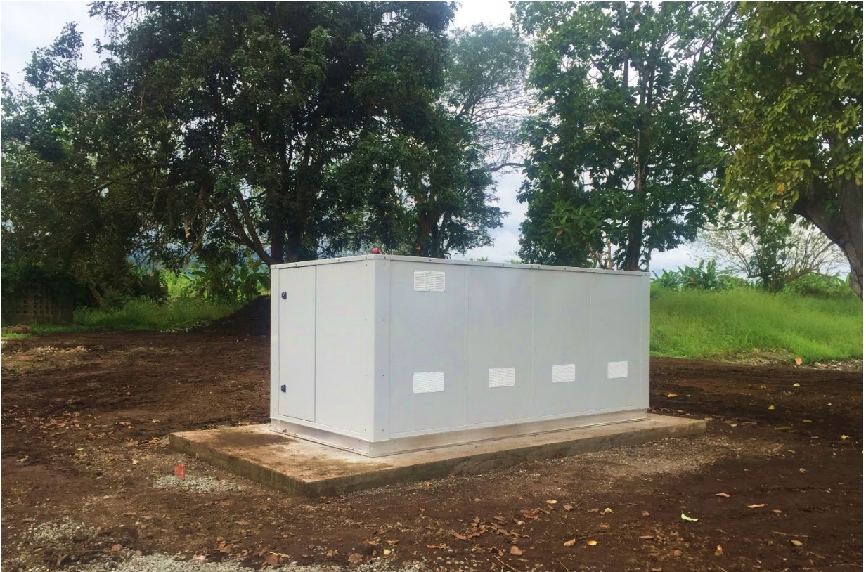
Figure 27 – The Control Room was designed to withstand the tropical climate and constructed out of powder coated steel.
