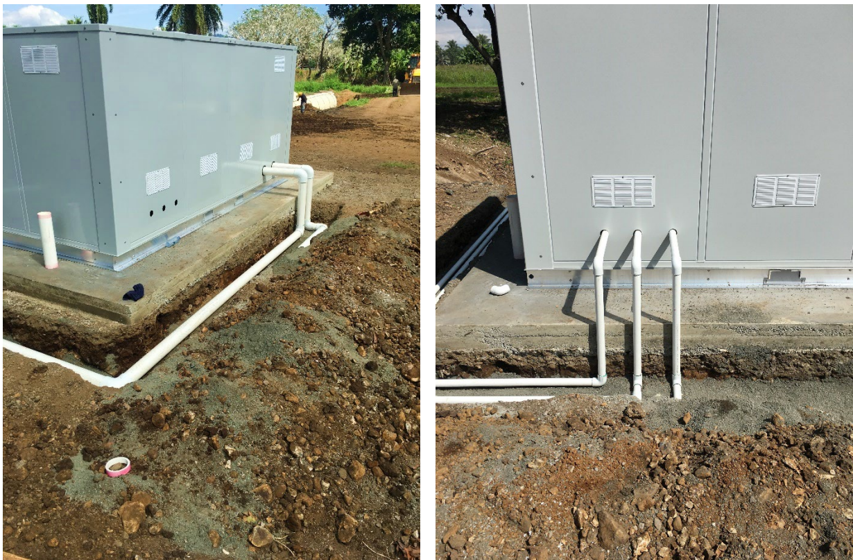
Figure 20 – Every aspect of the infrastructure is designed to ensure a quick and problem free installation onsite.
