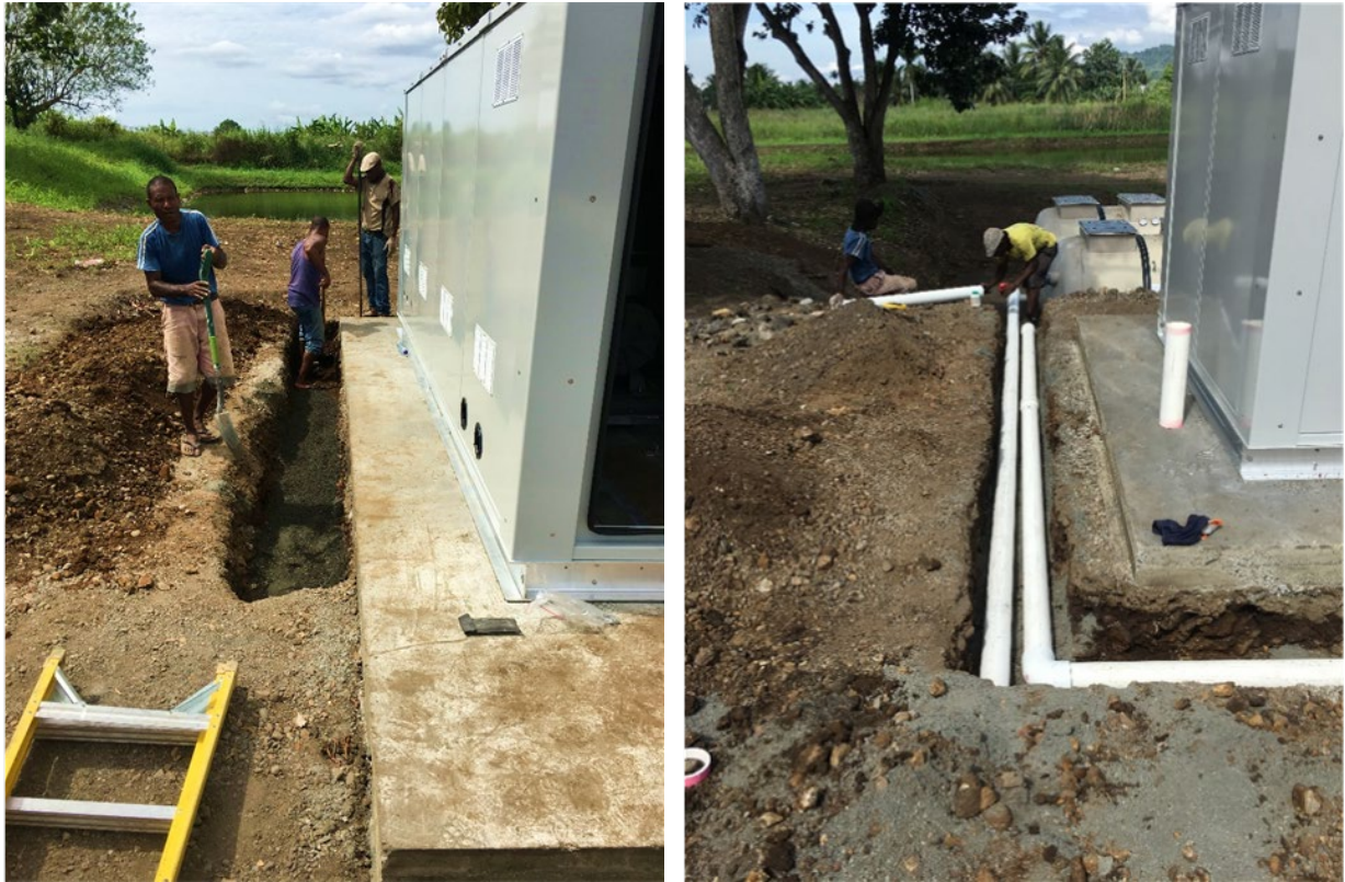
Figure 19 – Connection of the Control Room to the Kubota STP was completed with assistance from local trades.
