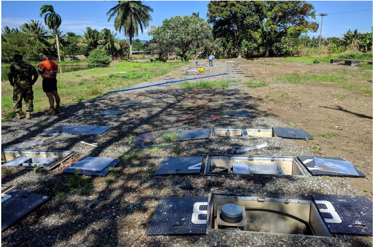
Figure 32 – The inspection lids allow access to the separate chambers of each STP module.
