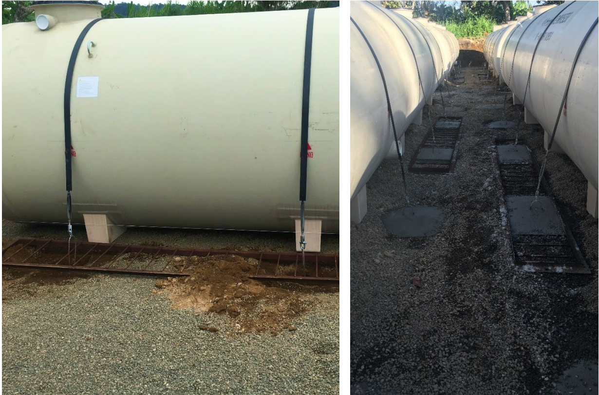
Figure 15 – STP modules anchored in position to prevent movement during extreme weather conditions.
