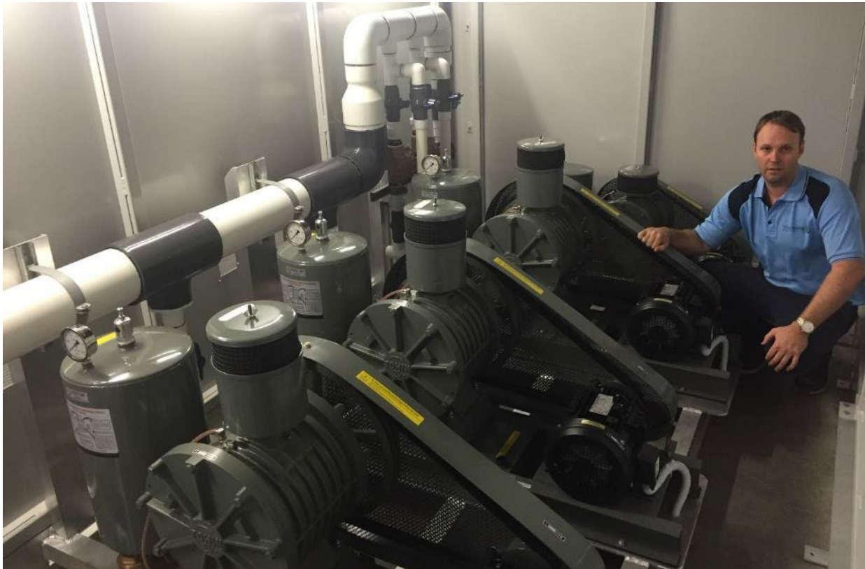
Figure 8 - Blower assembly and manufacture completed in Australia before shipping to the site.
