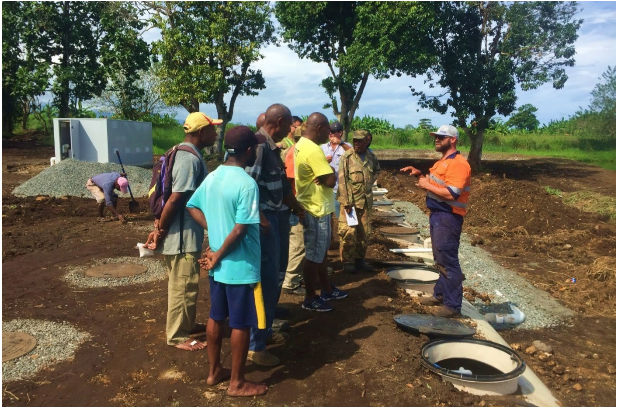
Figure 23 – All aspects of the STP that may require day to day maintenance are explained to ensure safety of onsite personnel, encourage and sense of ownership and responsibility for end users and guarantee continuity of service.
