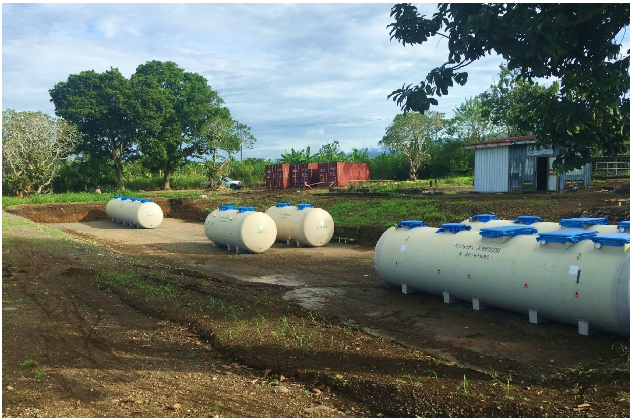
Figure 12 – The Kubota STP modules were installed in a treatment chain to specific design parameters.
