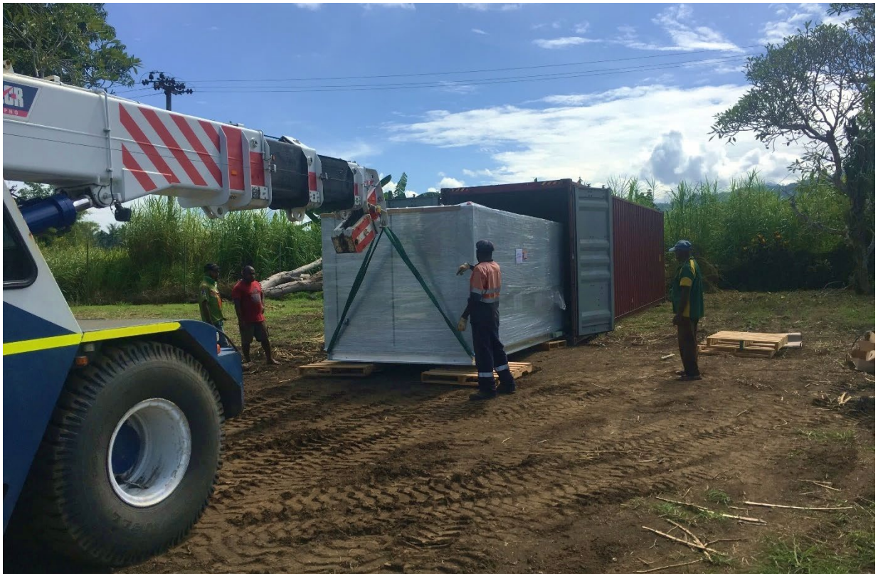
Figure 18 – Control Room and components were premanufactured in Australia and shipped to site.
