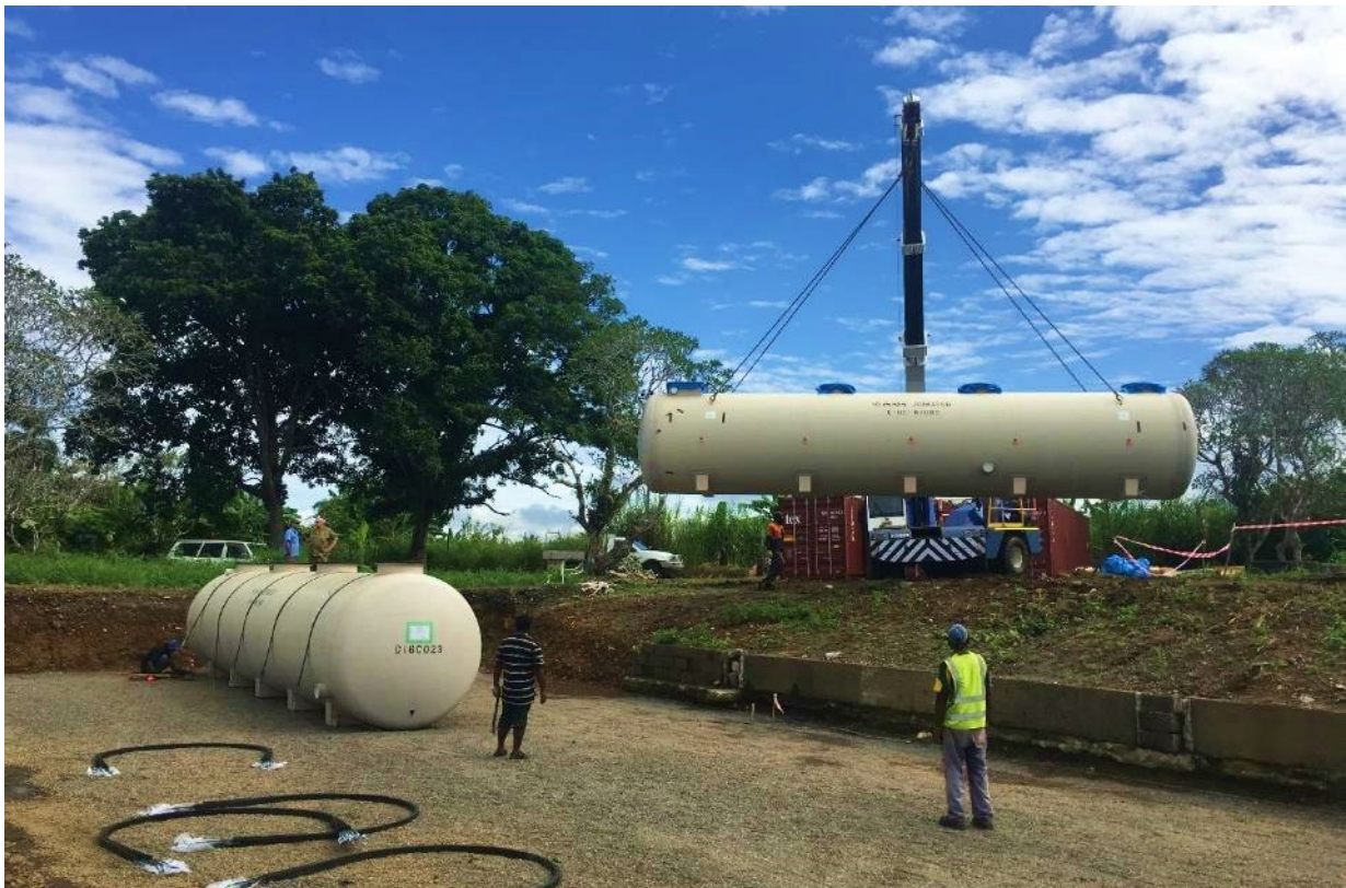
Figure 10 - The ground for installation was pre prepared to the specifications provided by True Water.
