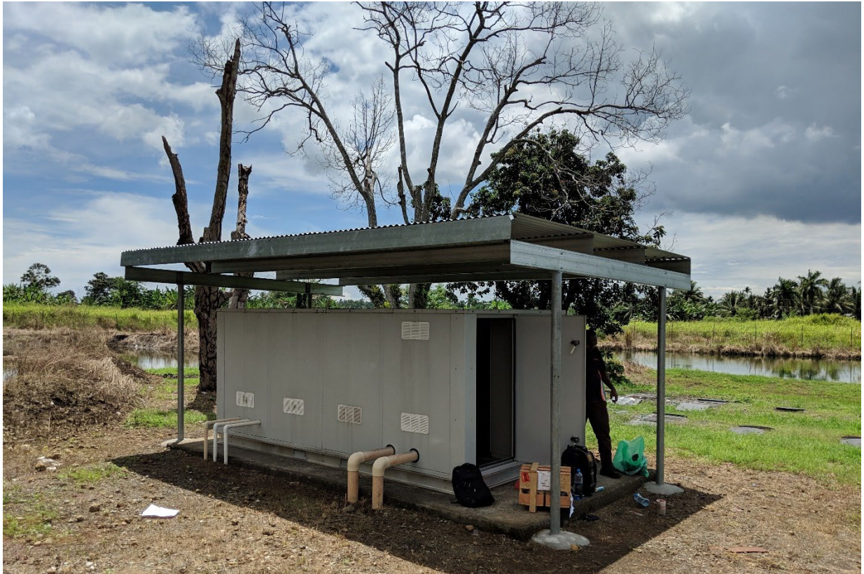
Figure 30 – The blowers and control panel undergoing a routine inspection as part of the asset management program.
