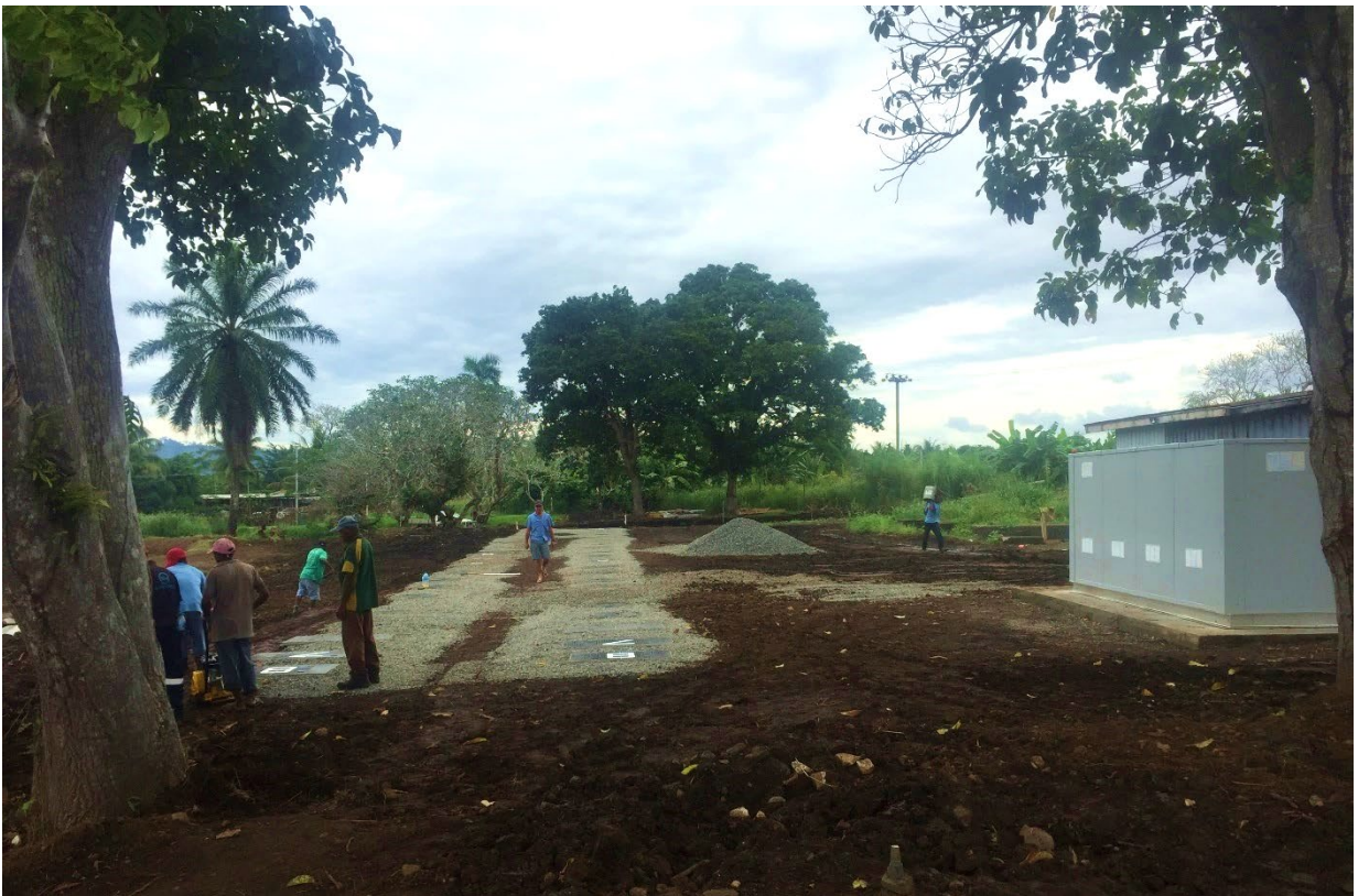
Figure 28 – Top dressing of the STP compound with gravel to aid in surface water drainage.
