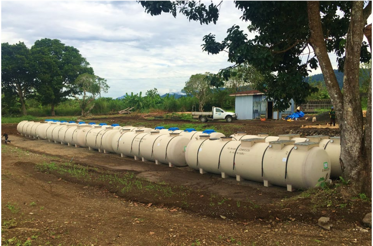
Figure 13 - Kubota STP in place and ready for the next stage of installation.
