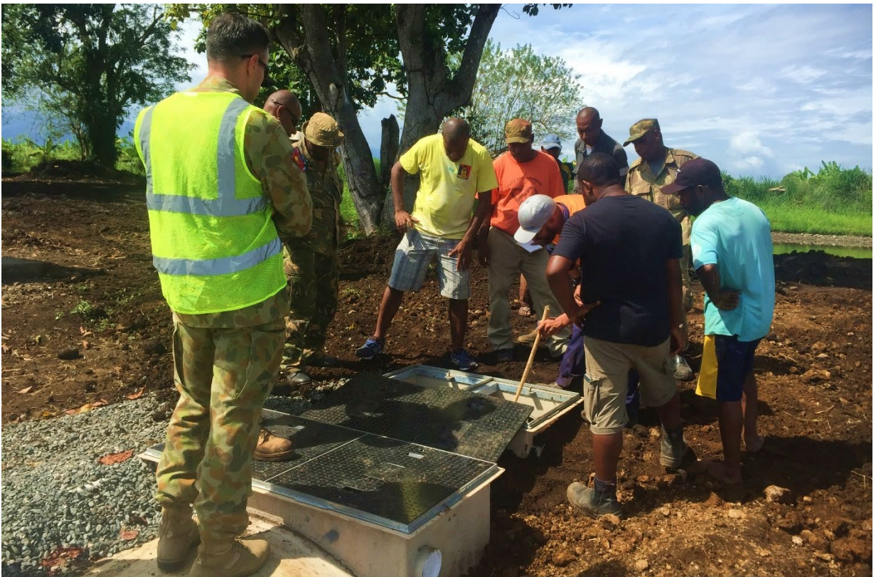
Figure 22 – Commissioning of the system was completed in conjunction with hands on training of onsite personnel.
