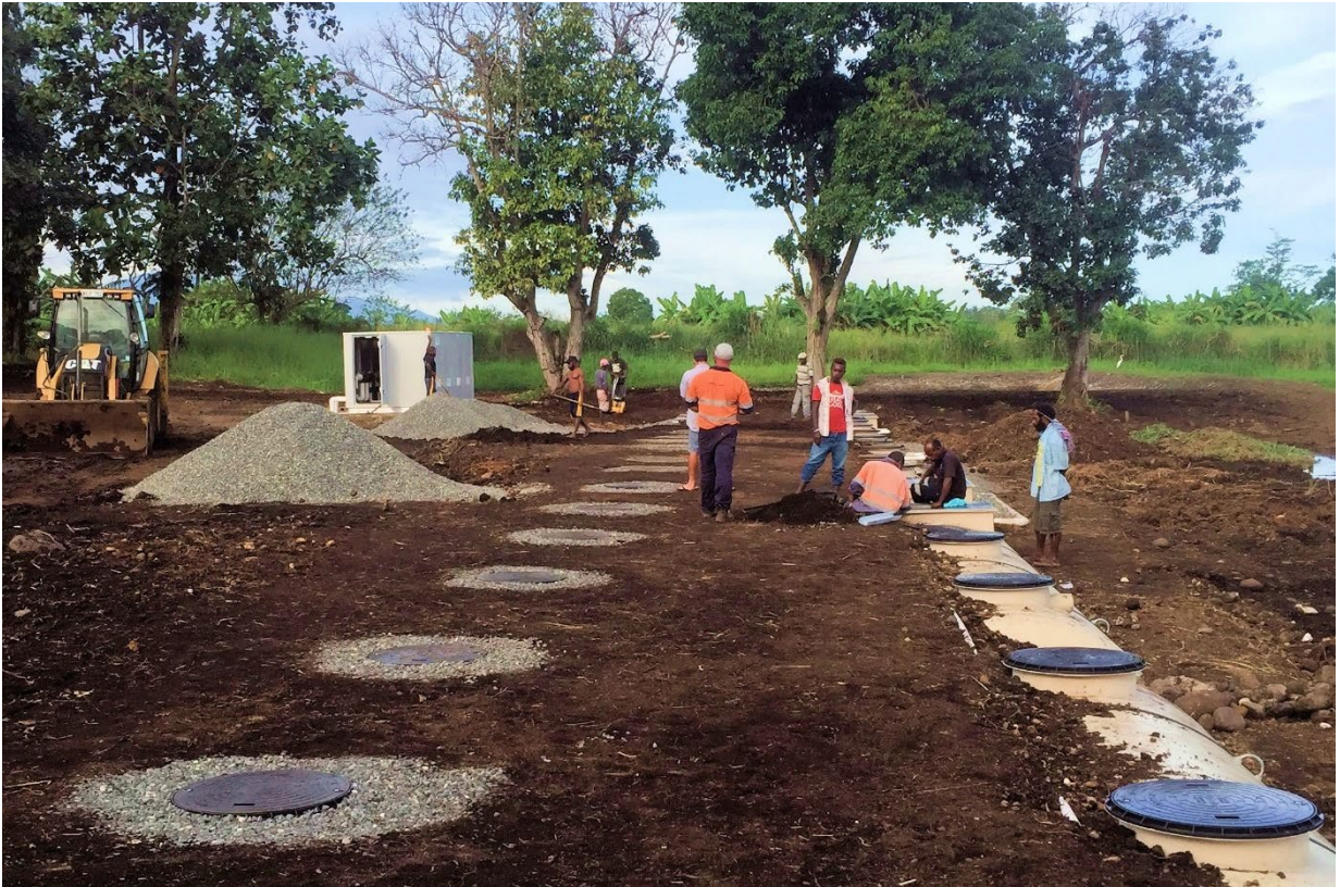
Figure 21 – Backfill of the system being completed with a gravel bed for adequate drainage around the inspection lids.
