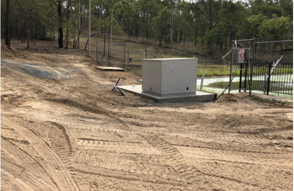
Figure 23 – Irrigation pump housing at Irrigation Pump Well
