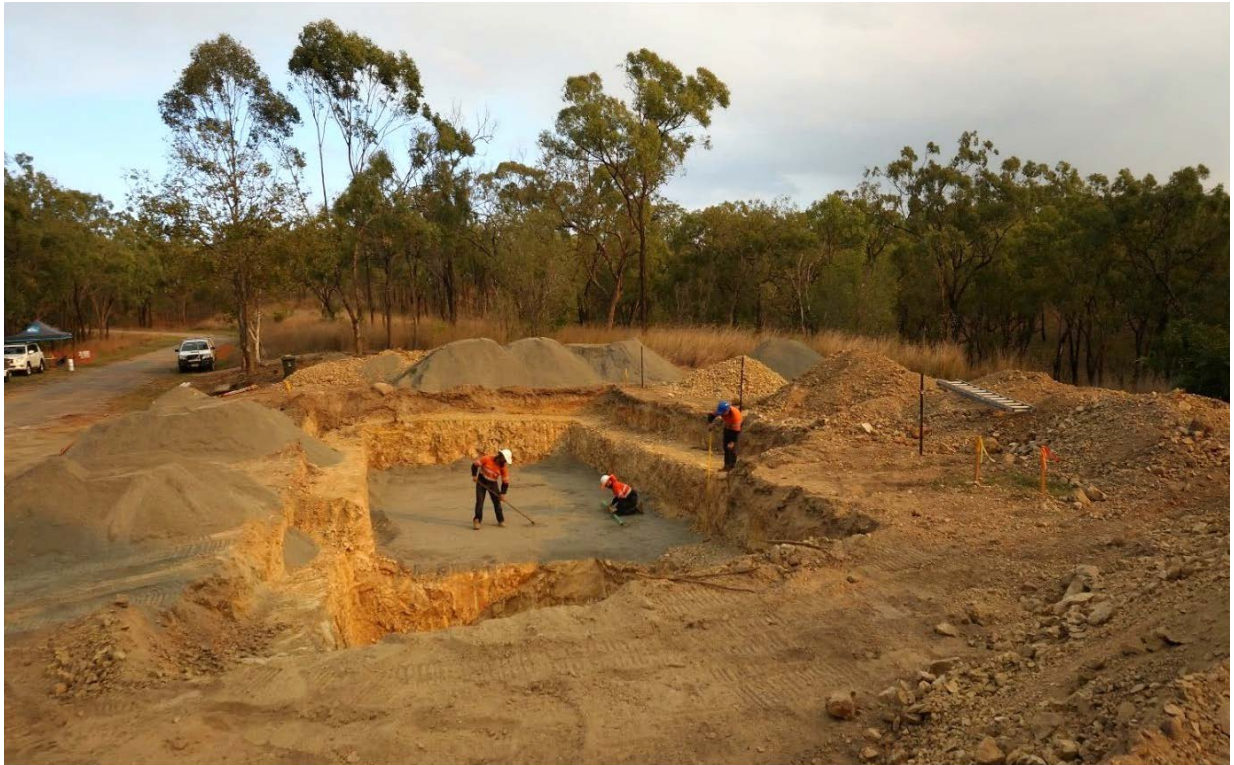
Figure 14 – Select material is levelled and compacted to form the foundation for the Kubota STP
