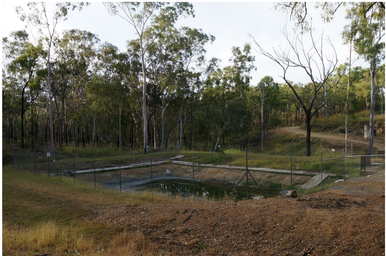
Figure 30 – Wet weather storage dam post clean out and lining with select material
