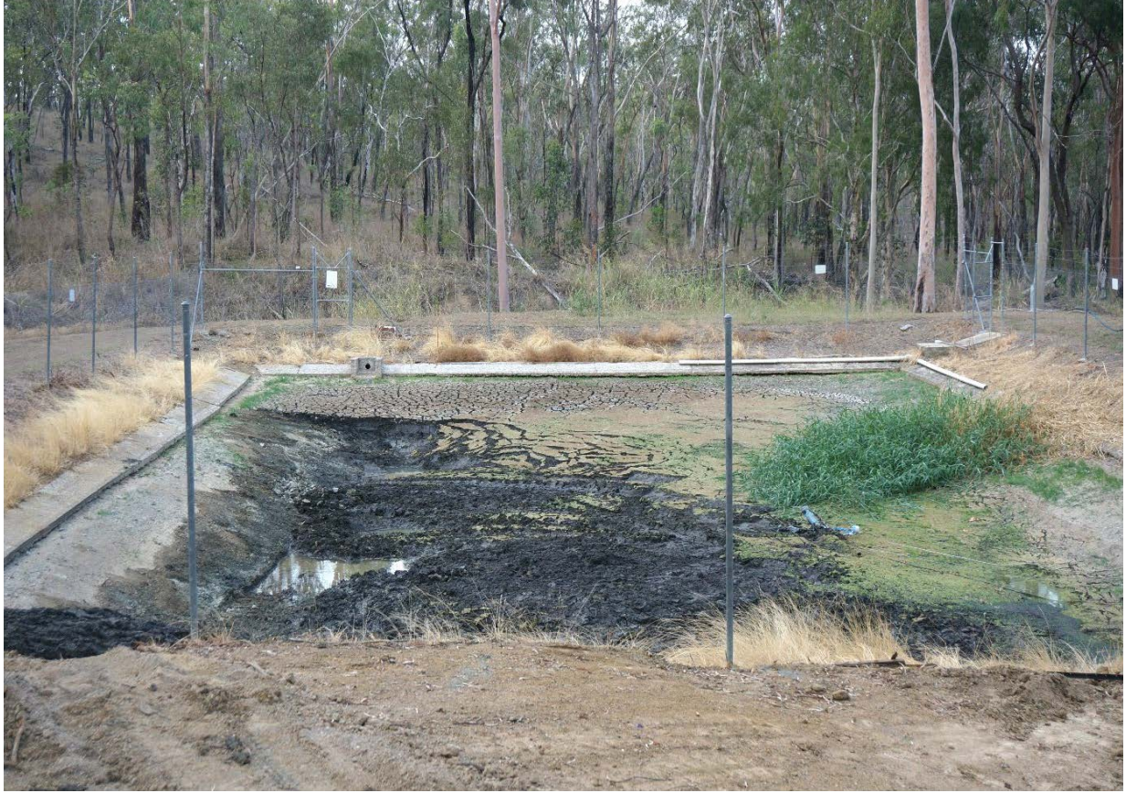
Figure 29 – Wet weather storage dam mid clean out, included removal of liquid waste and sludge
